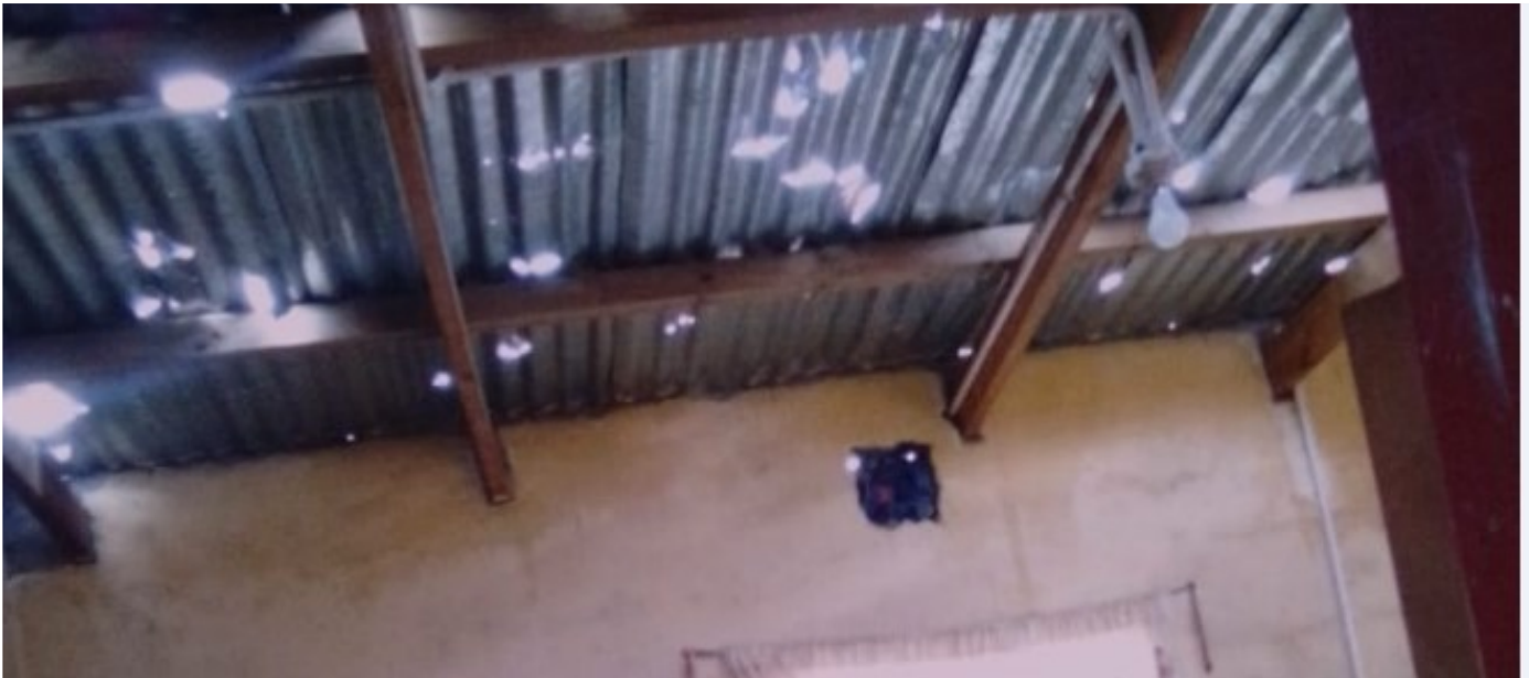
Roof destroyed by hailstones, as assessed by BERCS
